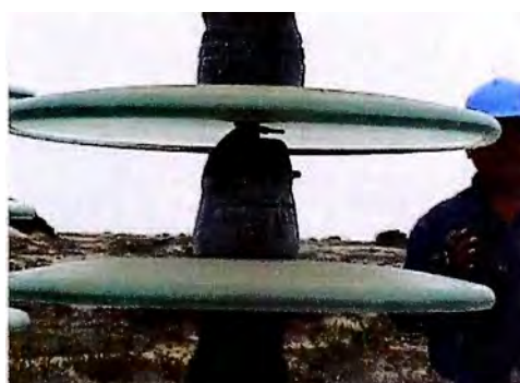
Foto 10A: Insulator # C125-4 – lee side
