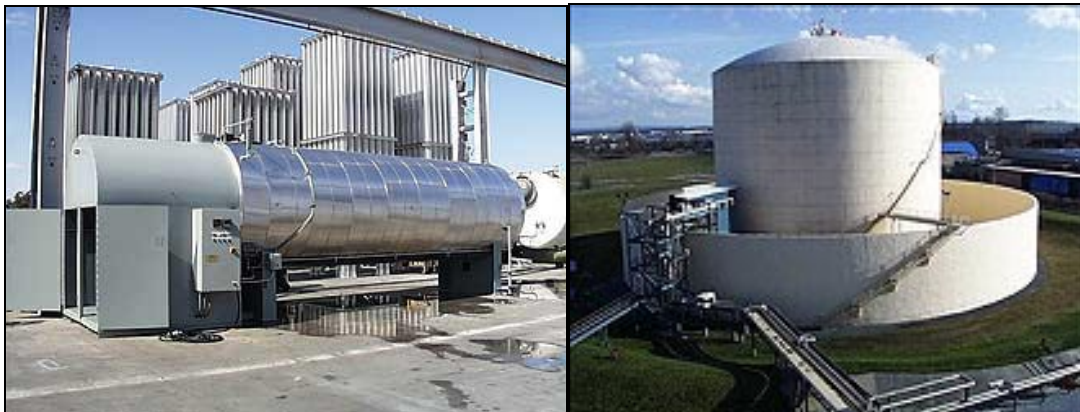
Figura N° 7: Planta de Peak Shaving
