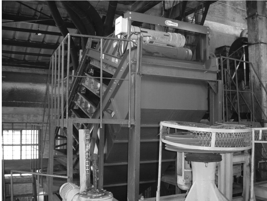
Figure 7: Stack Sizer in Operation at LaiWu Iron Mine, China
