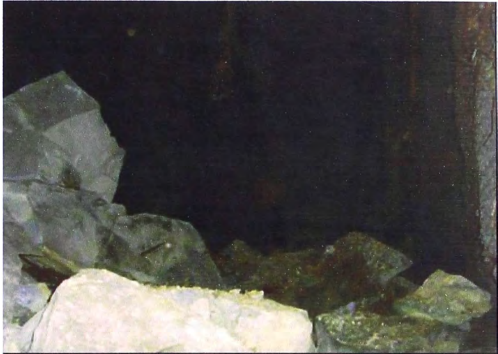
FIG No 5-4 By pass derrumbado
