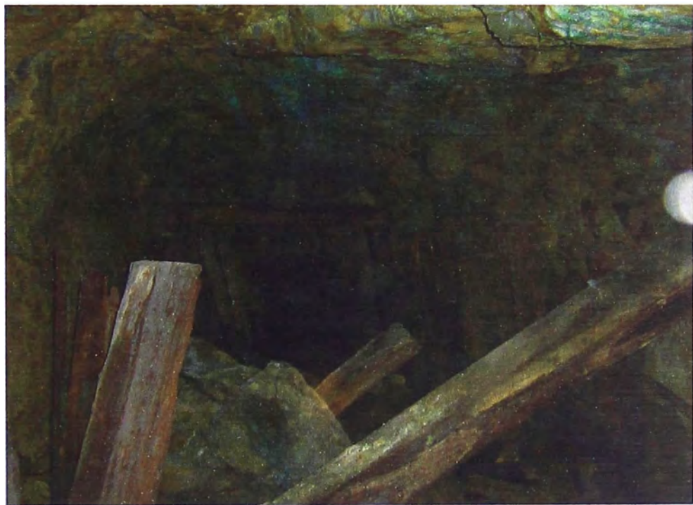
FIG No5-5 By pass derrumbado
