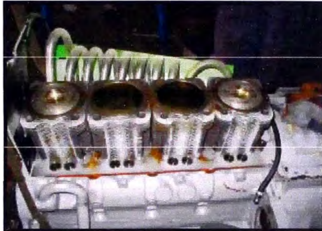
Fig. 2.8: Motor Diesel (Repetidora Acchi – Ayacucho)
