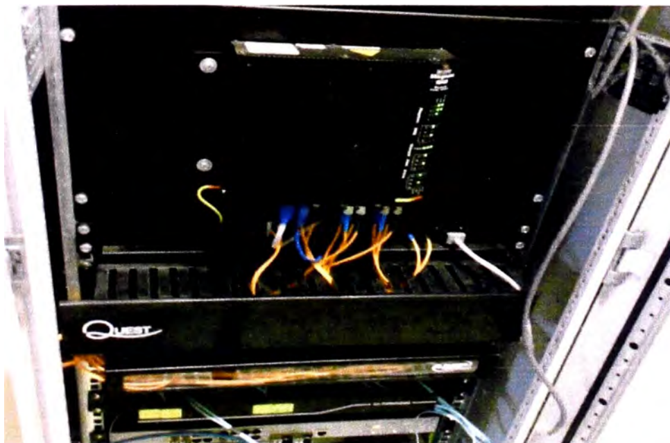
Figura 5.7: Switch y routers
