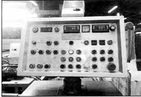
Figura 7.13 PANEL DE CONTROL PRINCIPAL
