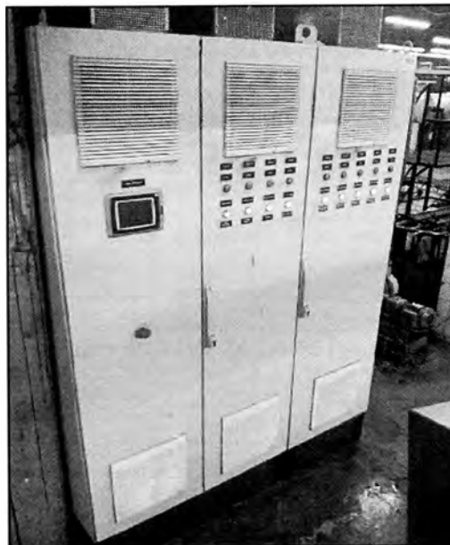
Figura 6.13: TABLERO DE CONTROL
