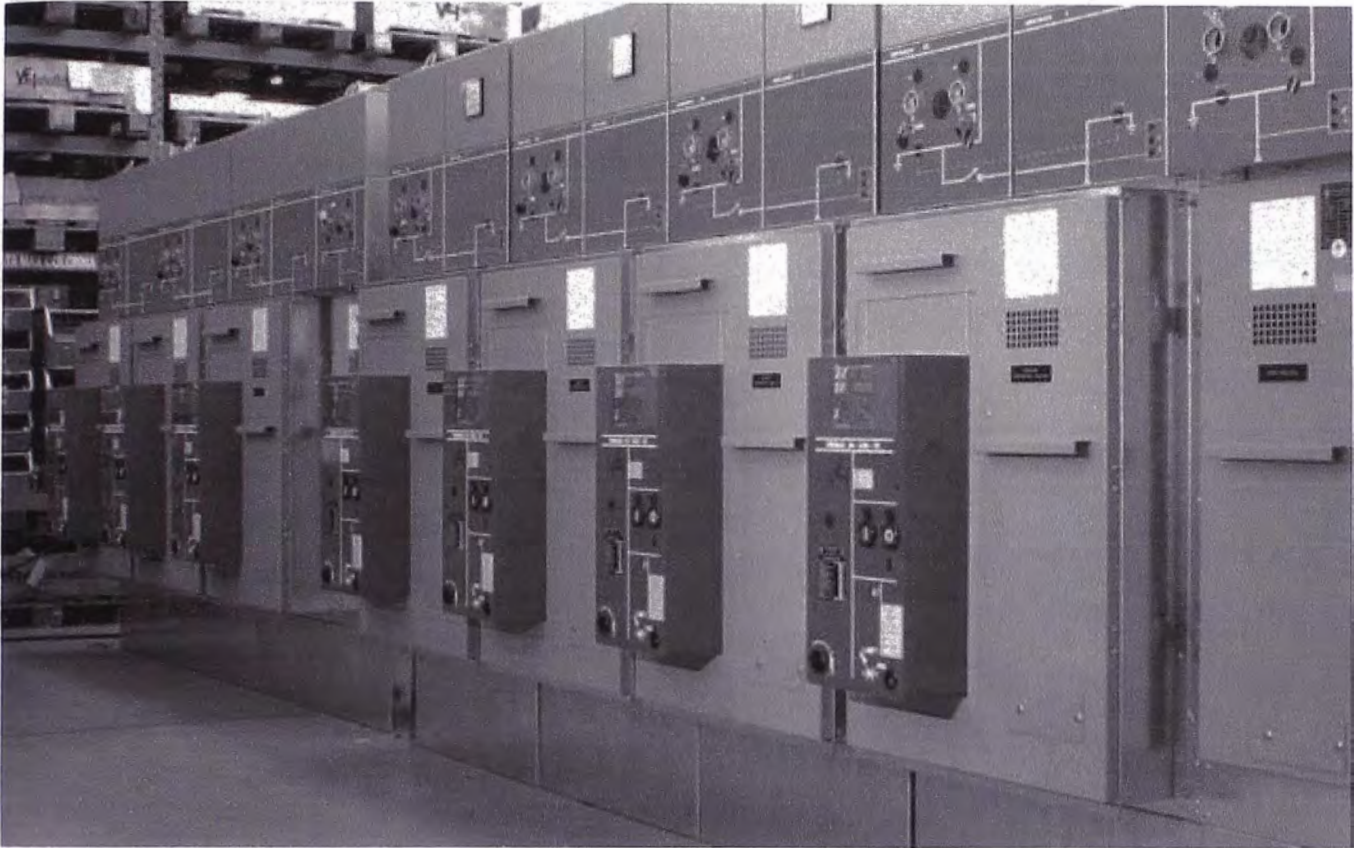
Quadro UNIFLUORC completo di rele' ed interruttori isolati in gas SF 6 (VEIGAS) UNIFLUORC switchboard equipped with relay and circuit breaker insulated with SF 6 gas (VEIGAS)
