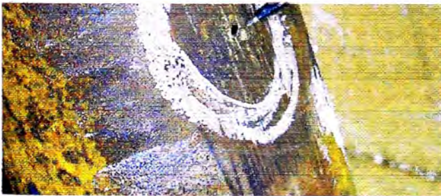
Figure 3 - Pinhole Caused a Leak
