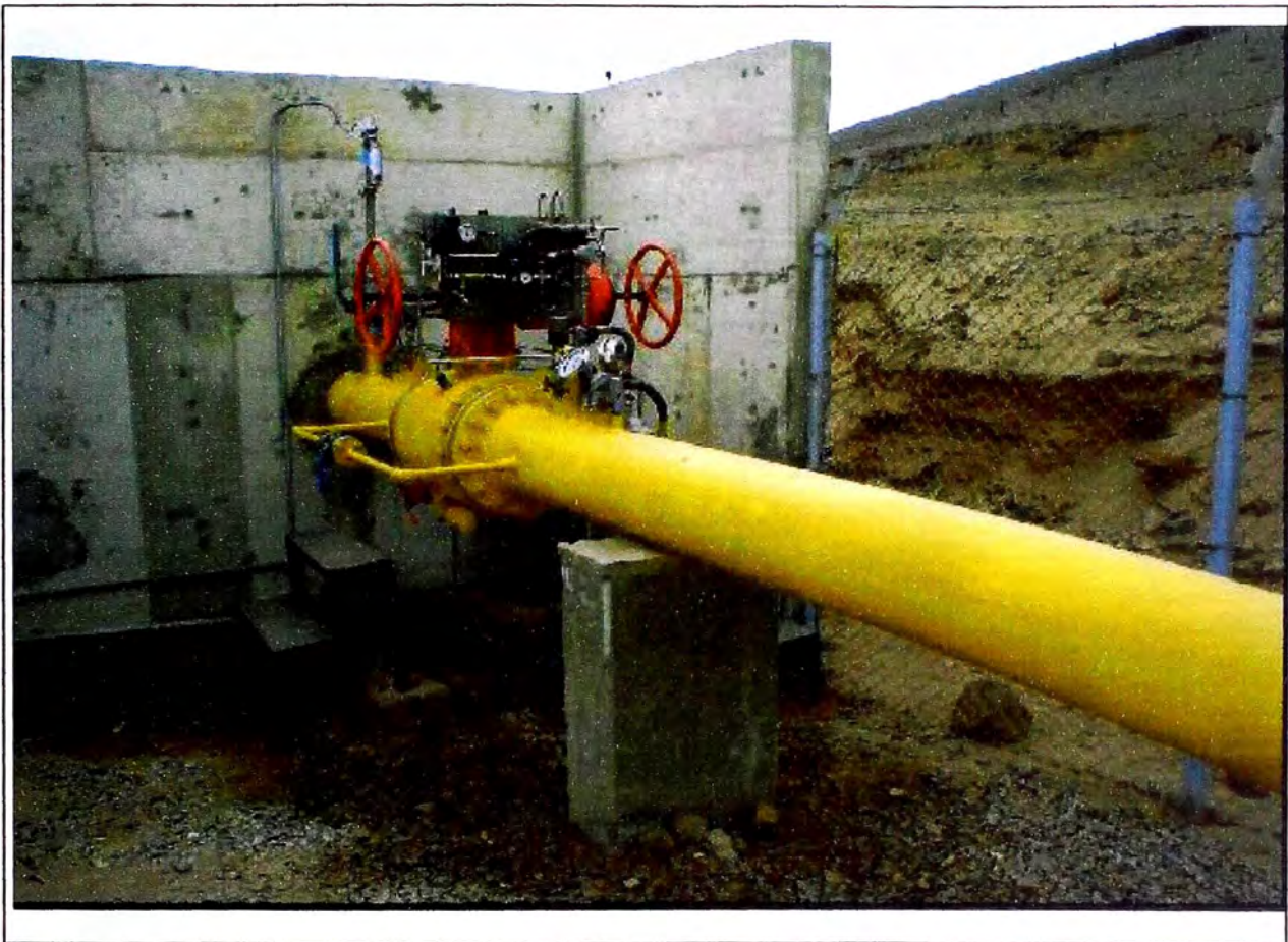
Figura 17: Suministro principal de gas natural
