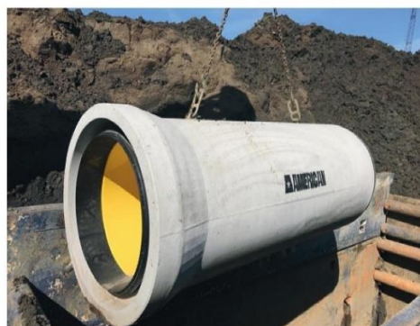
American Perfect Pipe is installed in Nebraska. A corrosion-protected flexible pipe system is produced immediately after the pipe has been installed.
