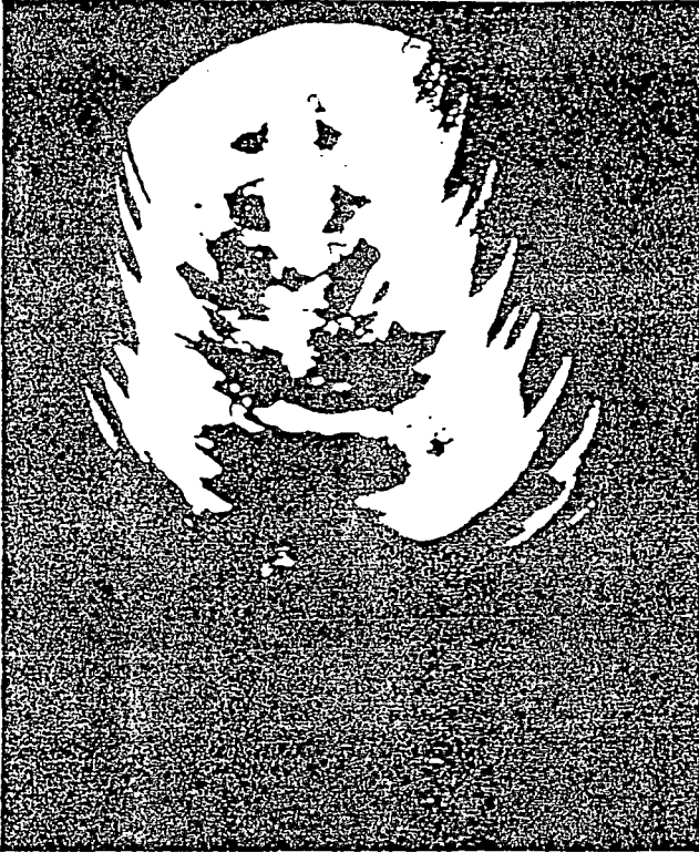
Fig. 2.4 — "Christmas tree" configuration of cavitation damage on a high-head tunnel surface
