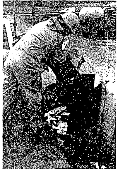
Fig. 9 No special equipment is needed to disperse Fibercon 19mm steel fibres in the concrete.
