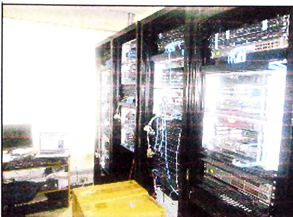
CENTRAL AVAYA CS 1000 CORE GERENCIA GENERAL
