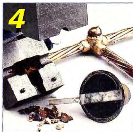
Open the mold and remove the expanded steel cup – no special disposal required
