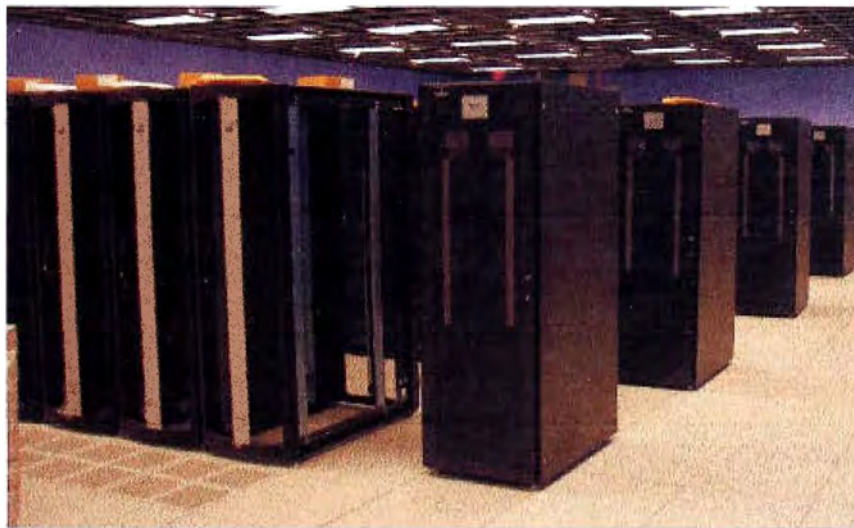
Figura 2.1 Data Center Principal de la empresa (Fuente: http://computerservicenow.wordpress.com/2011/07/21/obama-administration-shutting-down-800-data-centers/ )
